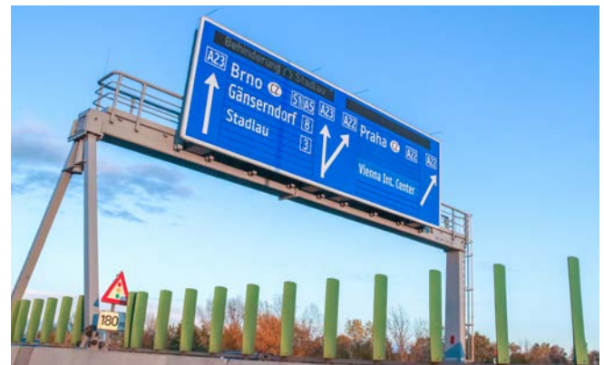
The gantries for the prism-type variable message signs were fitted with catwalks for maintenance.
